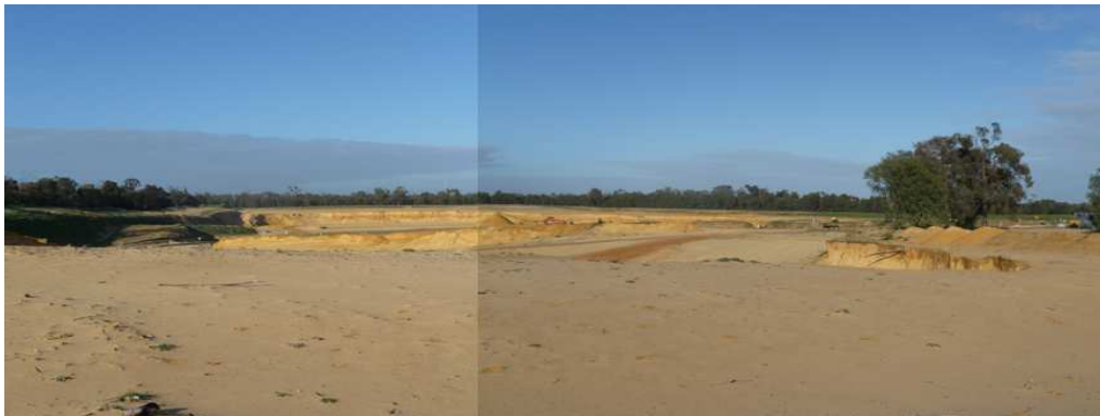
Plate 2 - Top of active extraction area (Lot 4 Runnymede extraction activities in central background) showing scraped top soil stockpiles to the right.
